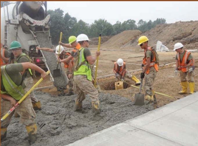
Marine Corps Reservists pouring the second Helipad. Photo courtesy of the JTF Summit Staff
