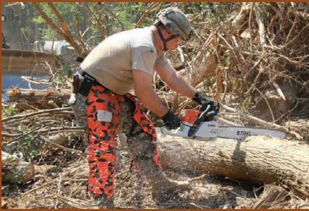
A Soldier from the 276th Engineer Battalion uses a chain saw to clear an access road into a planned Virginia Civil War Site. Soldiers from several Virginia National Guard units worked together on this IRT project as part of their annual training. Photo by Cotton Puryear, Virginia Department of Military Affairs
