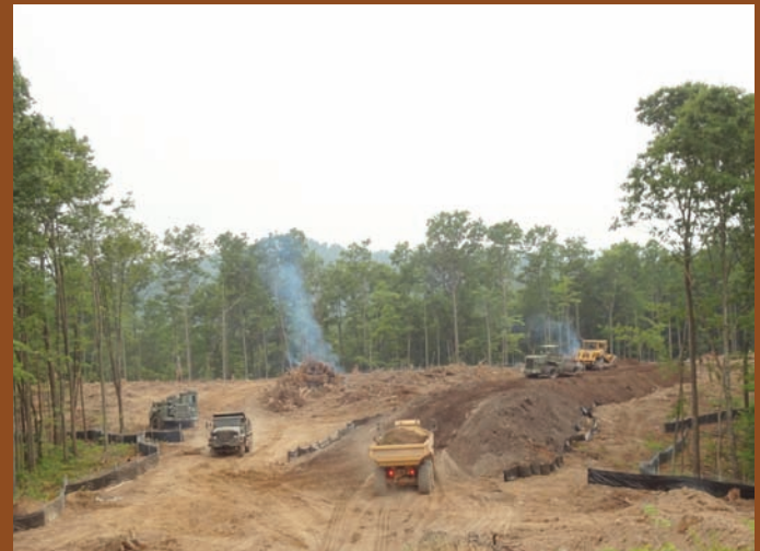
Staging Location of Top Soil for the Presidential Helipad. Photo courtesy of the JTF Summit Staff
